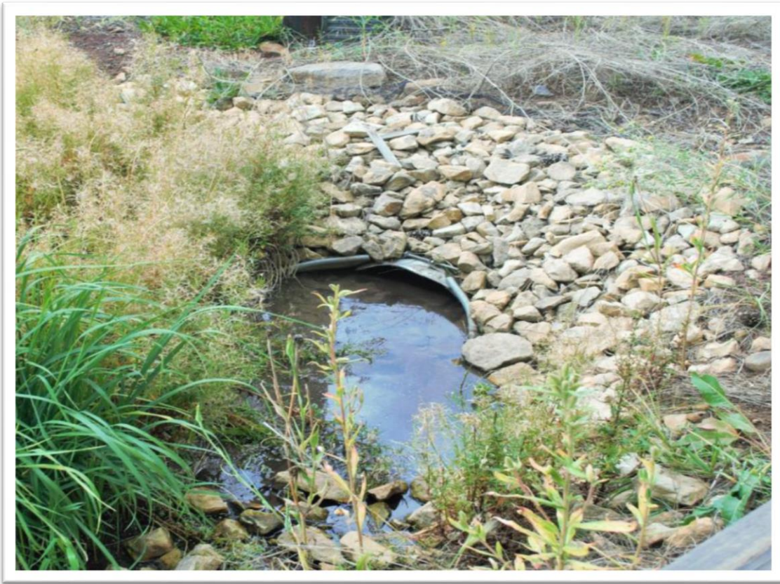
Figure 2: Clogged Culvert in Coyote Springs reach
